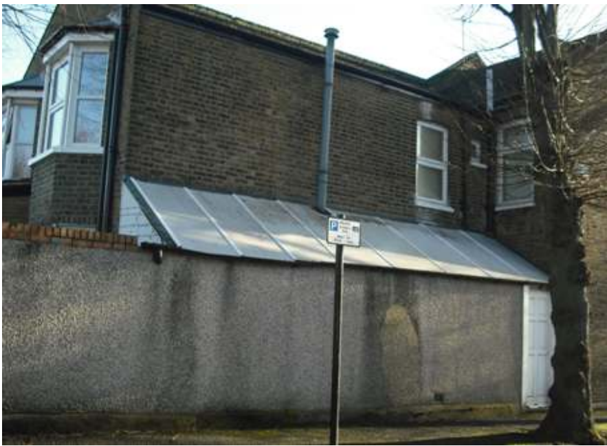
This is another example of a single story side extension at 39 Leybourne road E11 3BS
